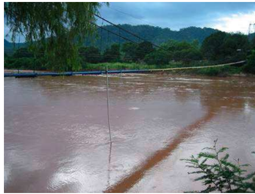
Figure : Installation of the limnimeter in the Rio Parapeti. The pressure probe is inserted into the pole.
